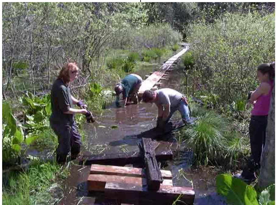
Bog Bridge Construction on the M-M Trail (photo by Pat Fletcher AMC)
